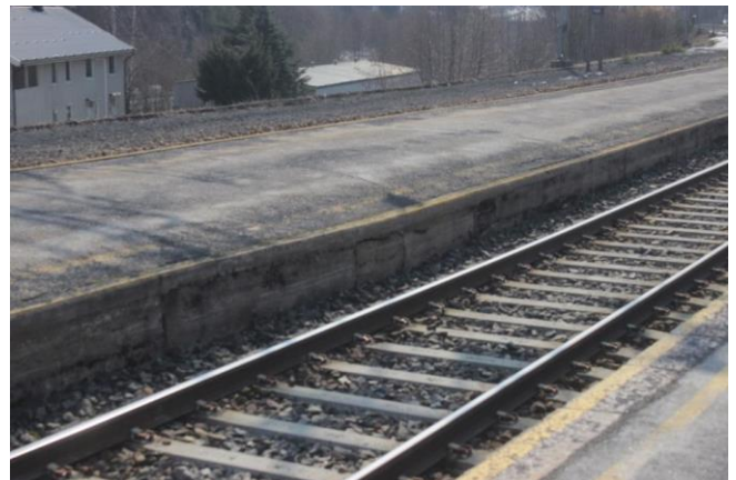
Platform at Drangedal needing significant work
